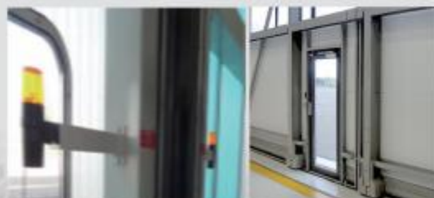
个人安全门及车门信号系统 Personal safety door and door signal system
